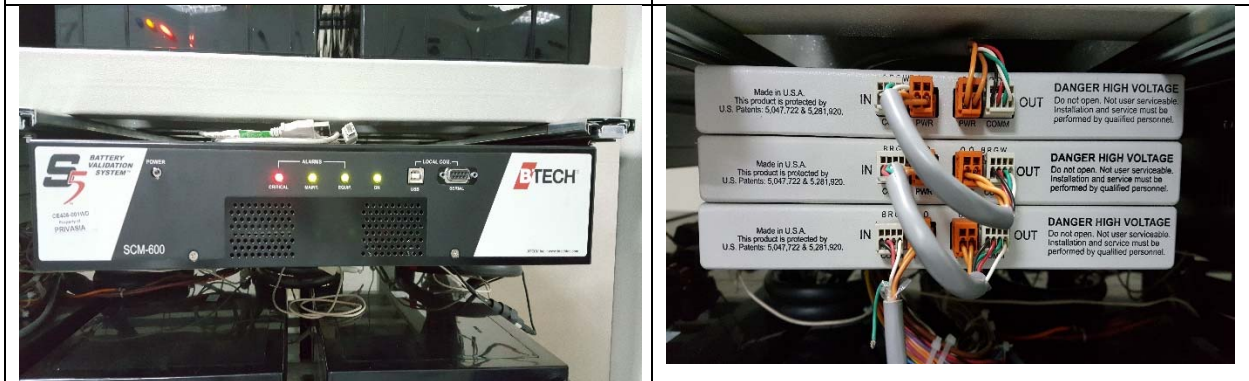
Photo 3& 4: User existing UPS battery monitoring system (Brand: BTECH SCM-600)
