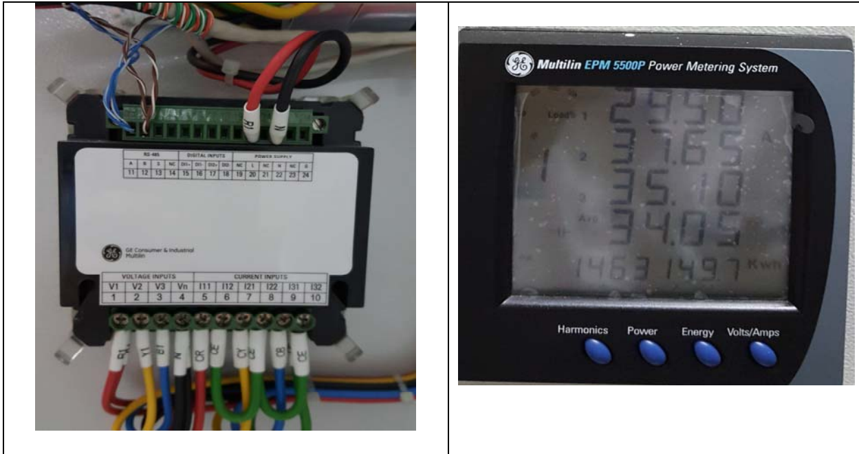
Photo 1& 2: EPM 5500P Power Metering System, generate RS 485 input for AC-SB 1 and AC-SB 2.
